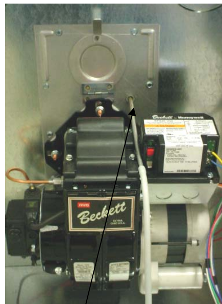
Over-fire draft access port.
